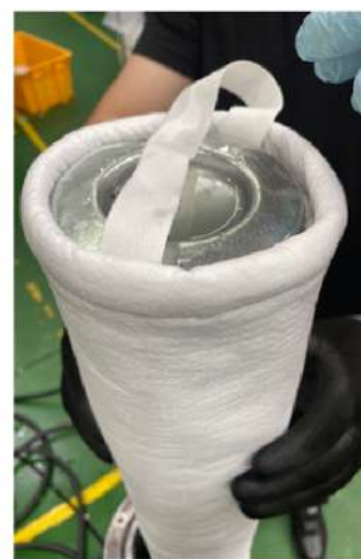
Removal of band filter from particle filter housing
